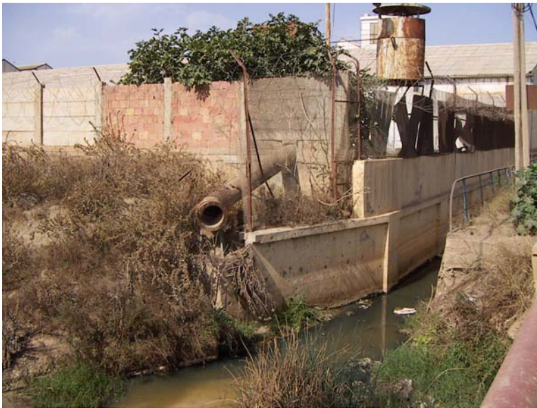
Plate 6: Wastewater is discharged directly into the river streams without appropriate treatment.
